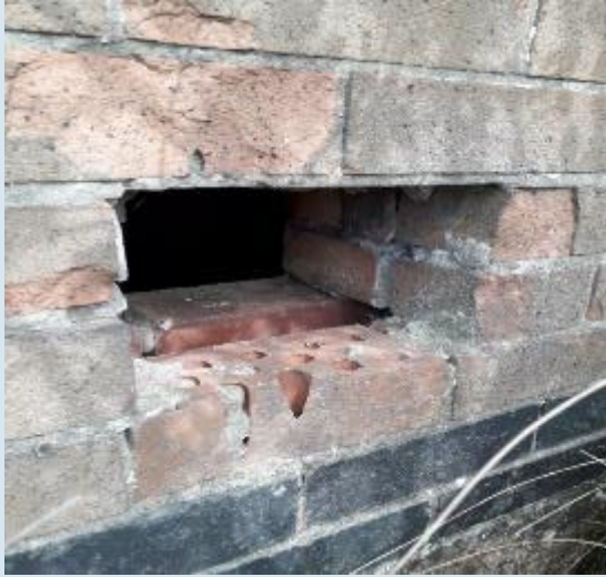
Photograph 9 – Missing brick in Building 8
