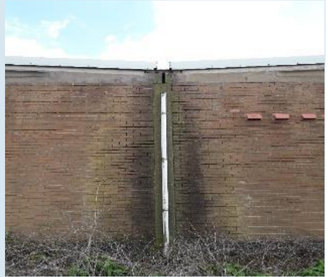
Photograph 10 – Missing concrete in Building 5
